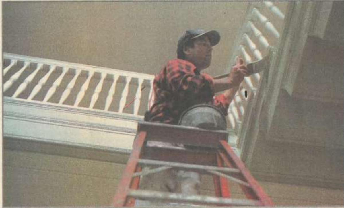
■ Tom Campbell of Chapman Painting and Decorating, Middletown, paints the main stairway. The paints and finishes are as close a match as possible to the mansion's decorative scheme in the 1930s.
