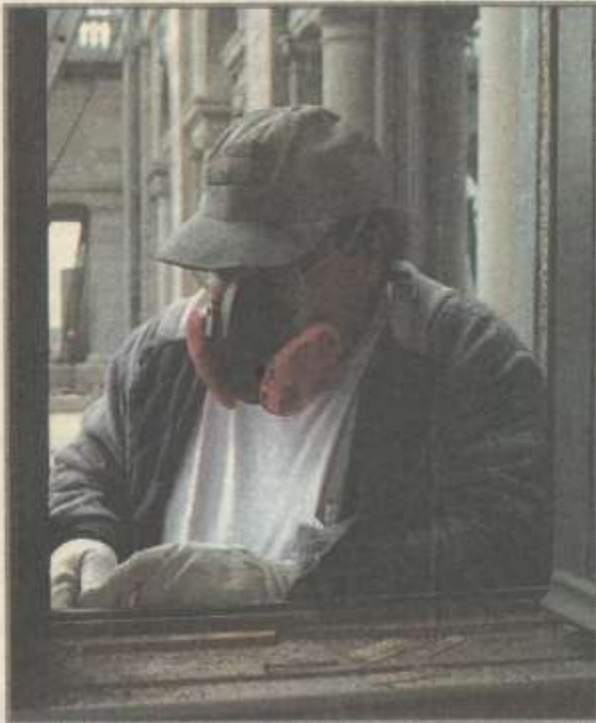
■ Moe Cushman of Kronenberger and Sons, Middletown, prepares a window to be painted
