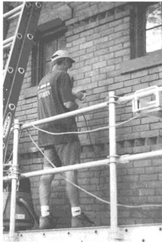
The restoration crew removes mortar from the east side of the Carriage House to prepare for the repointing of the bricks.
