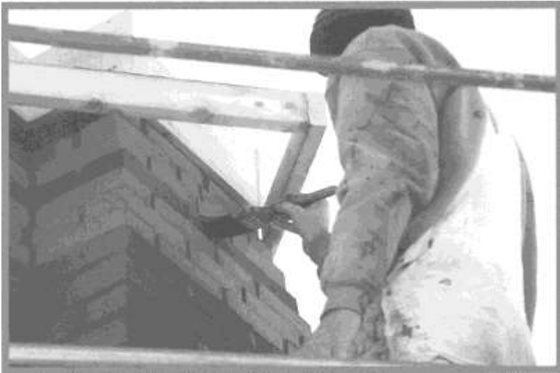
Craftsmen paint exterior bricks black and vermilion to match the original designs.
