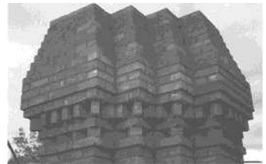
A newly rebuilt chimney before painting shows the complex patterning of brick in the original designs.
