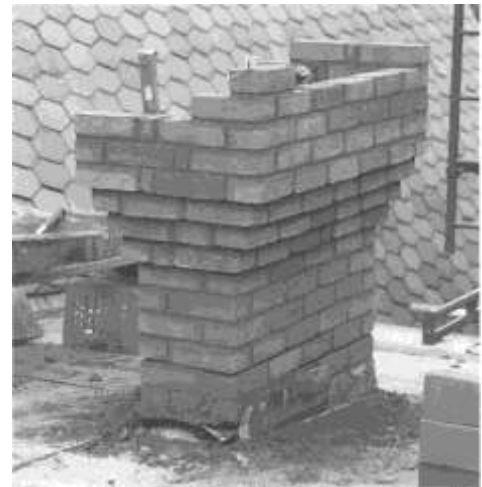
Each of the chimneys was torn down and rebuilt to replicate those seen in the Clemens-period images of The Mark Twain House
