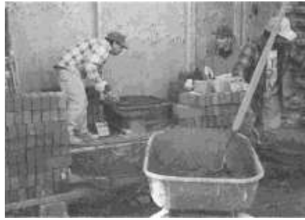
Bricklayers replaced the opening left by the removal of the doors with bricks carefully chosen to match the color of the original materials.
