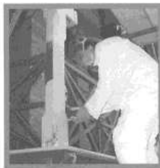
Ihor Budzinsky, a master carpenter from Kronenberger & Sons restoration firm, uses an epoxy solution to repair wooden supports on one of the porches (detail at right).
