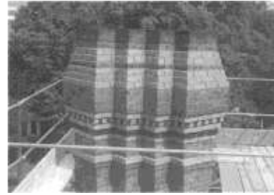
Before its restoration, a chimney on The Mark Twain House shows an earlier attempt to copy the original designs of the Clemens home. Through the enlargement of historic images by photo digitization, Curator Marianne Curling discovered that the original chimneys were more sculptural in quality.
