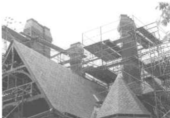
The Mark Twain House's restored chimneys appear at last as they originally were meant to be.
