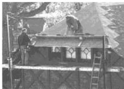
The restored slate roof of the carriage house was fitted with Yankee-style gutters. Made of wood and copper flashing, the gutters sit directly on the roof.
